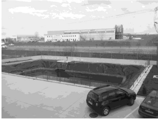
Fig. 2 Retention tank at Lebario Industrie. Bolentin Deal. Romania (authors' archive).
