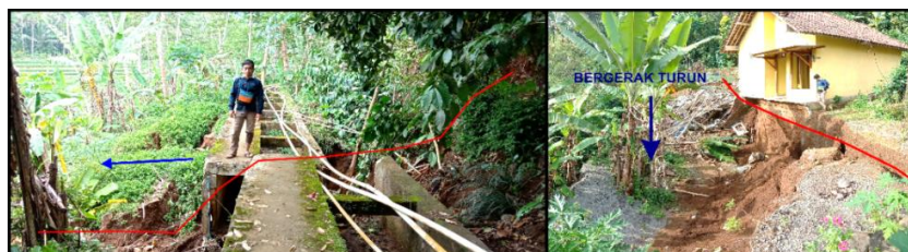
Fig. 9. Slope 7 (LR 7), and the direction of movement (blue arrow).
